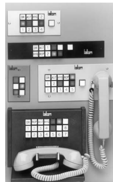
Figure 10-61. Communication system control panels. (Photo courtesy: Kelkom Systems, Redwood City, CA.)
