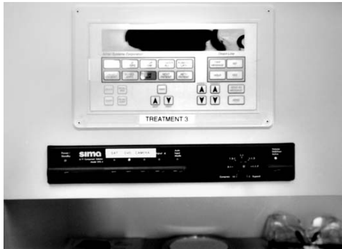
Figure 10-46. Communication system and AV control panel built into 12 o'clock wall. (AV consultant: Mr. Hookup, San Diego; Photographer: Jain Malkin.)
