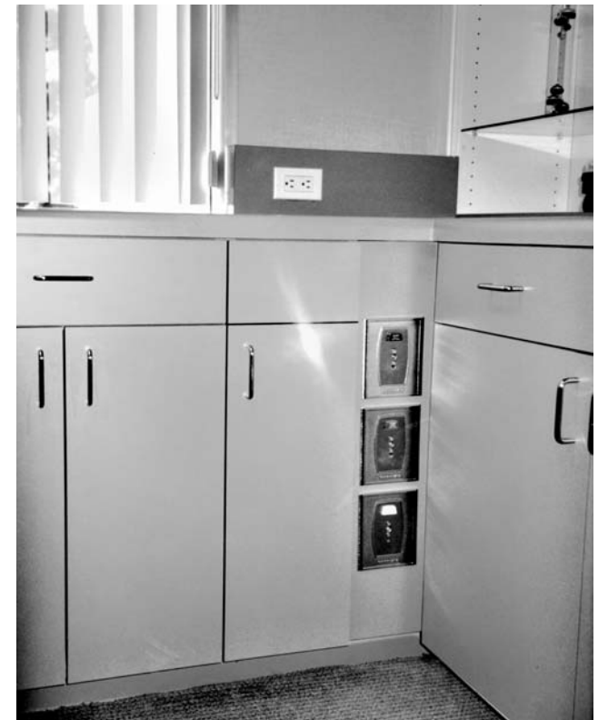
Figure 10-58. Outlets for medical gases at toe of dental chair, placed for convenience of anesthesiologist. (Photo courtesy: Cheryl Sheets, D.D.S.; Photographer: Jain Malkin.)
