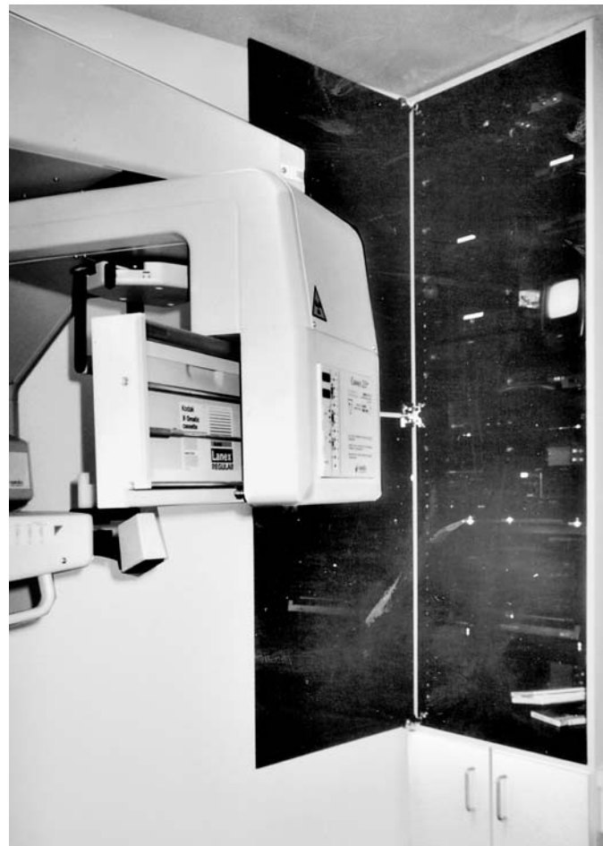
Figure 10-47. Central media station built into wall cabinet in X-ray alcove. (AV consultant: Mr. Hookup; Photographer: Jain Malkin.)
