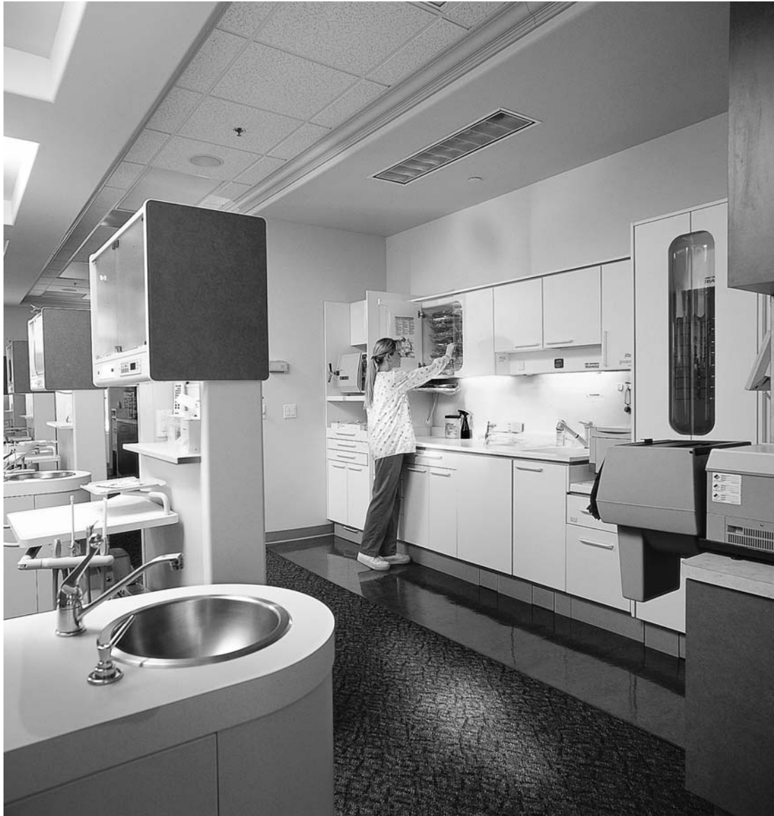
Figure 10-62. Triangle Furniture Systems, Inc. (Quebec, Canada) Steri-Center. (Photo courtesy: Patterson Dental Supply, Inc., St. Paul, MN.)
