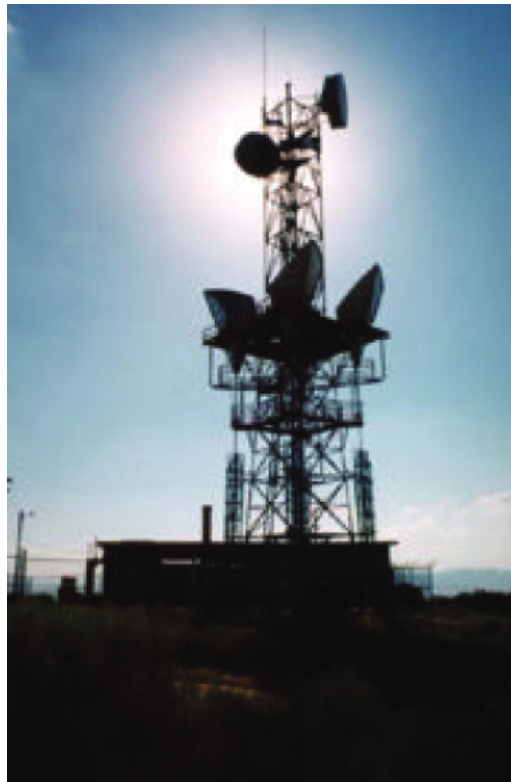
Figure 13.13 Microwave communication tower. (From www.wikipedia.com .)
