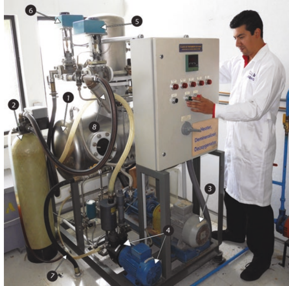
Fig. 5.17 Photograph of the water treatment plant (Wiegand GmbH, Ettlingen, Germany) used to deionize and degas the water of an HM3 lithotripter (Dornier MedTech GmbH, Wessling, Germany), showing (1) the degasser tank, (2) the deionization tank, (3) the degasser motor that pumps water to the tub, (4) the vacuum motor and the pump that creates vacuum in the degasser tank, (5) the mixing valve, (6) the input valve to the degasser tank, (7) the output to the tub, and (8) the water filter. (Photograph: F. Fernández)
