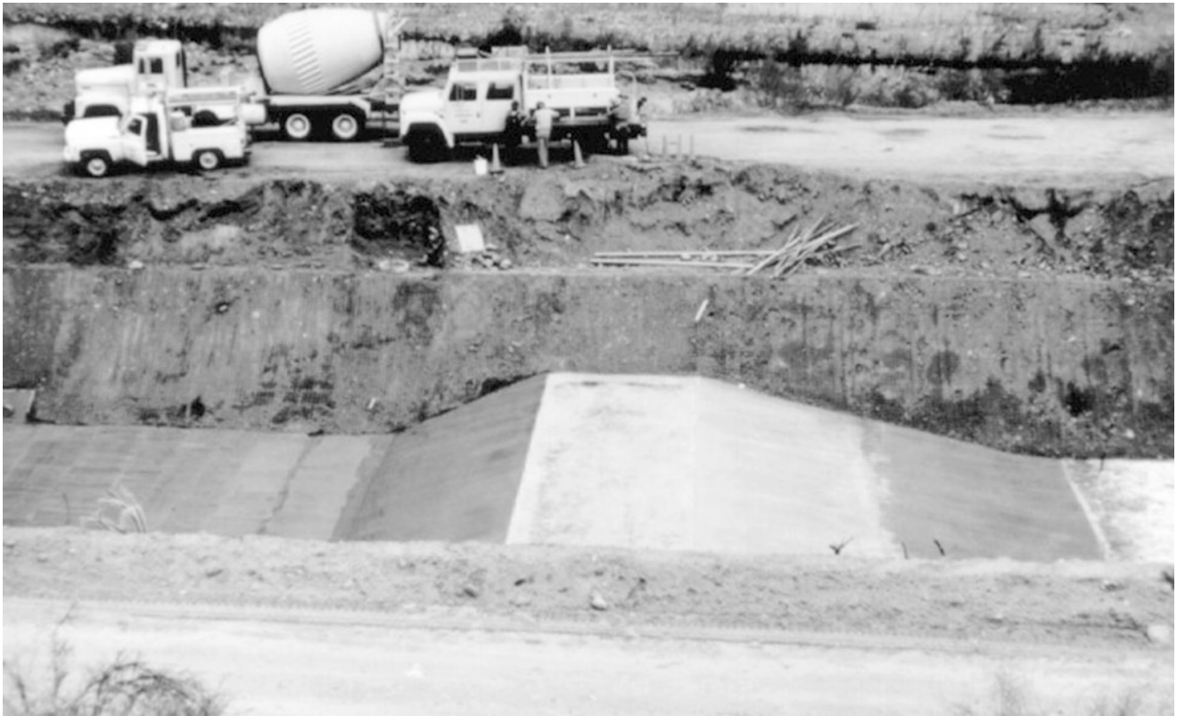
Fig. 11.26 Large long-throated flume under construction (Credit U.S. Water Conservation Laboratory, Phoenix, Arizona)
