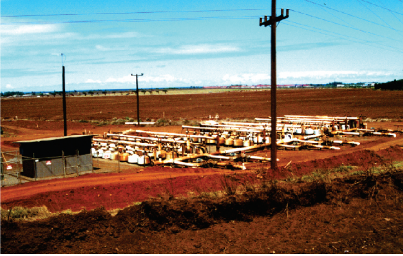
Figure 1.9. Large complex of sand media filters used to filter sugarcane mill wastewater for microirrigation, Maui, Hawaii, USA. Photo courtesy of Freddie Lamm, Kansas State University.
