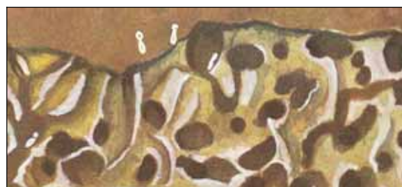
Fig. 118. Timber damaged by termites. Paper thin walls between runways creating a honeycomb. Photo©NSW Dept of Industry and Investment (E.H.Zeck).
