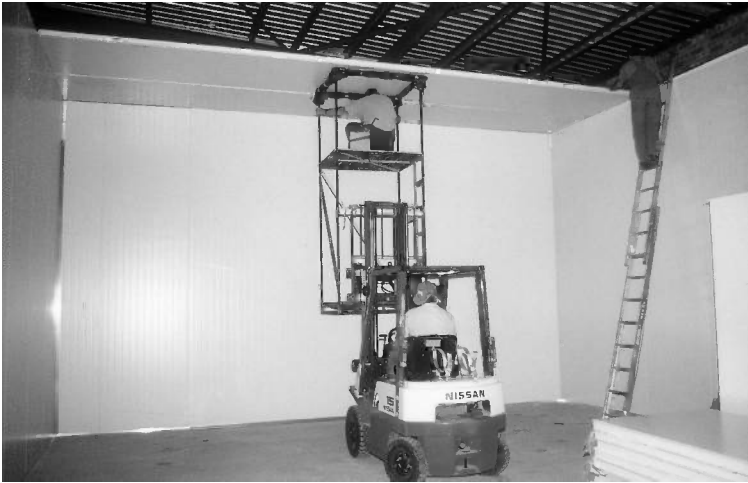
Figure 7.3 A modern cool room being constructed using metal-clad panels insulated with polystyrene. A Colorbond® finish has been applied to the panels to facilitate cleaning. All joints and entry points for electrical cables and plumbing are sealed with waterproof silicone mastic to prevent water entering the insulation.
