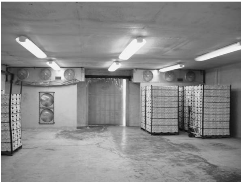
Fig. 5.2 Forced-air pre-cooling units in a refrigerated room.
