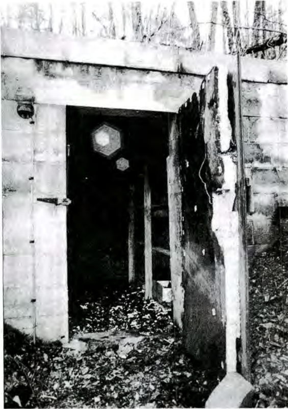
The insulated door of the Knier cellar with hasp. Note the light to the left of the door.
