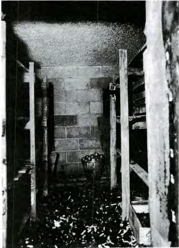
The Knier root cellar has storage shelves on each side of the central aisle, and a gravel-covered dirt floor.
