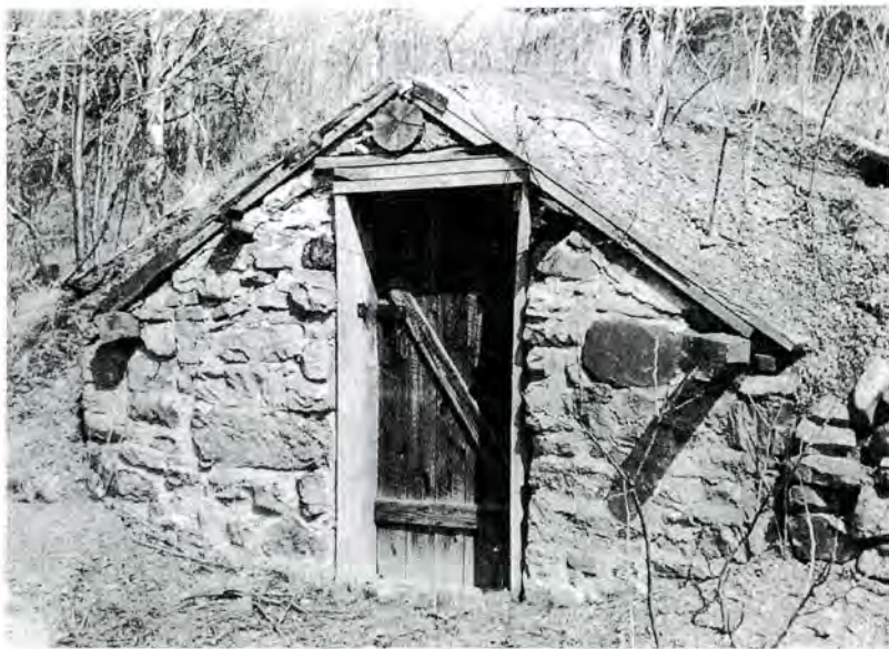
This is the old root cellar in Buffalo Valley, Pennsylvania, that got us started collecting root cellars.
