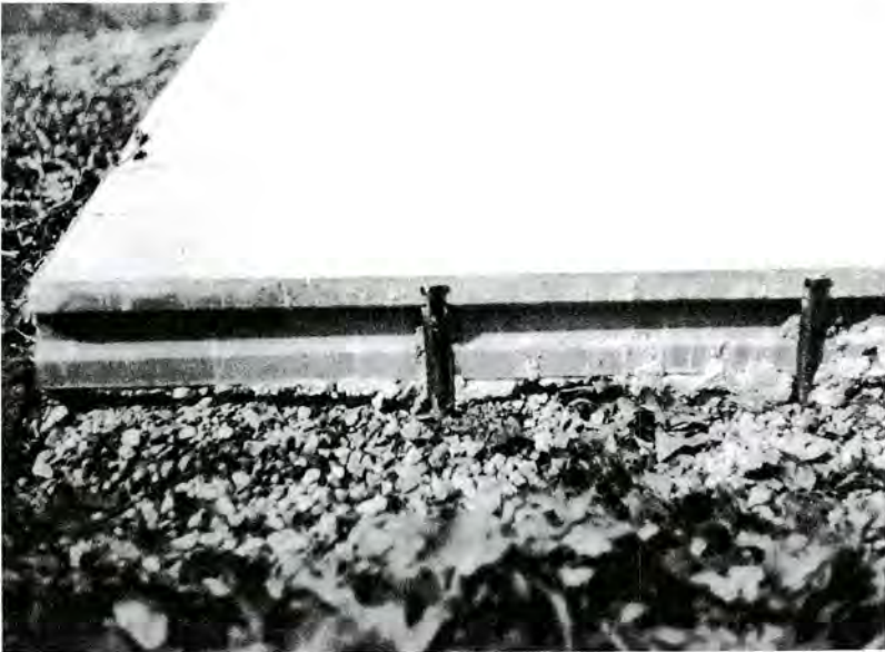
The Gravers' metal expansion joint.
