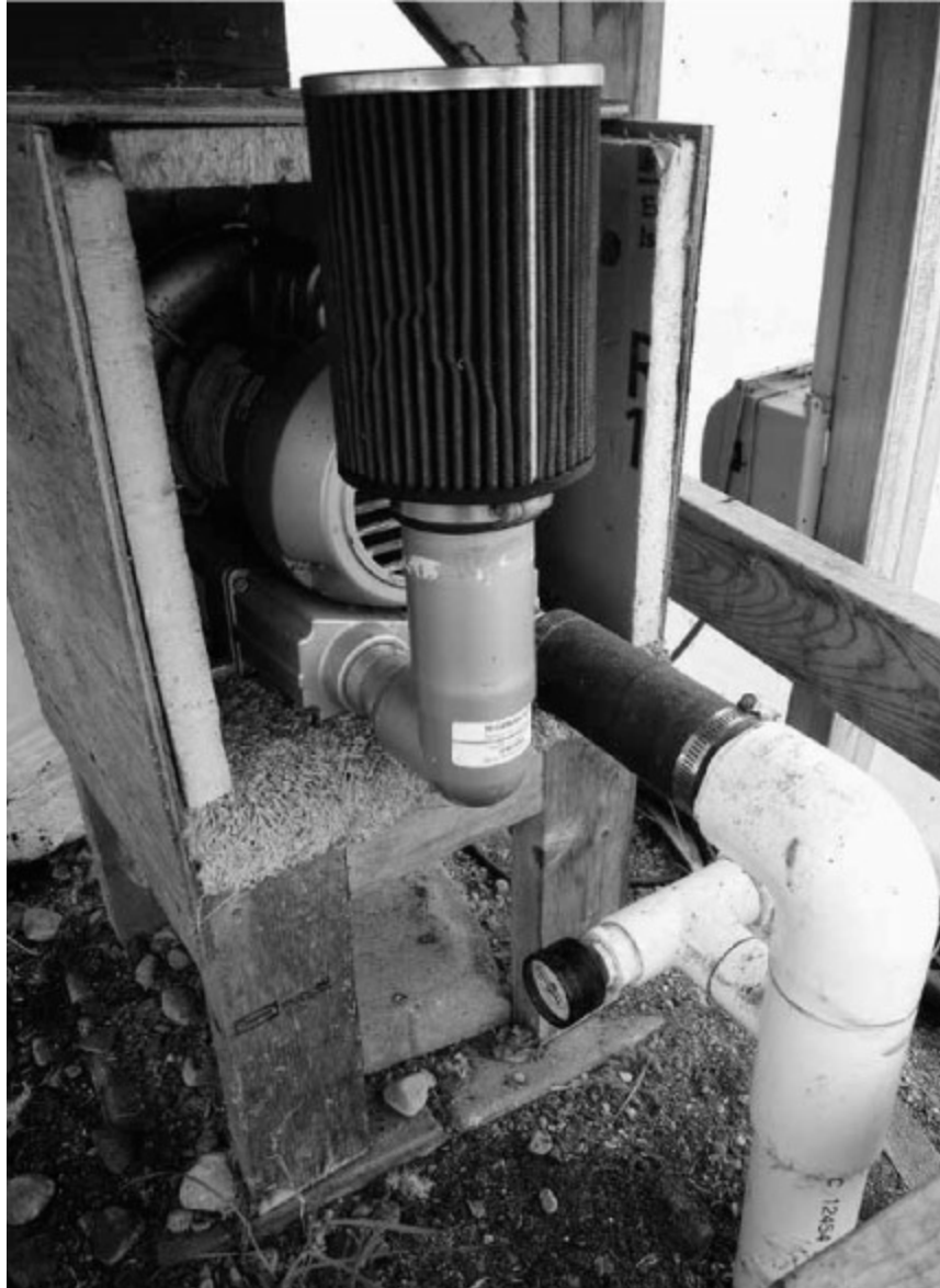
Aeration blower in sound-dampening box with front of box removed.
