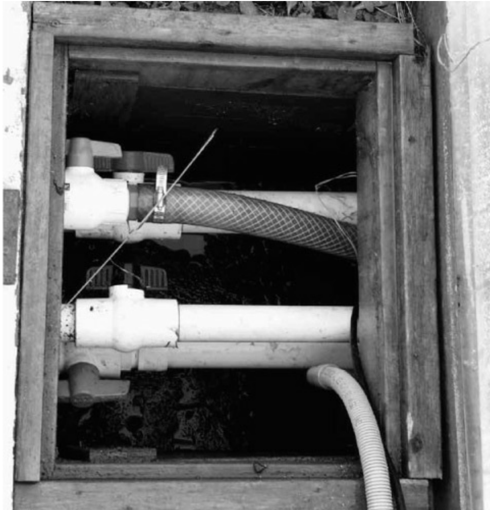
Heat pump and cistern valve service box.
