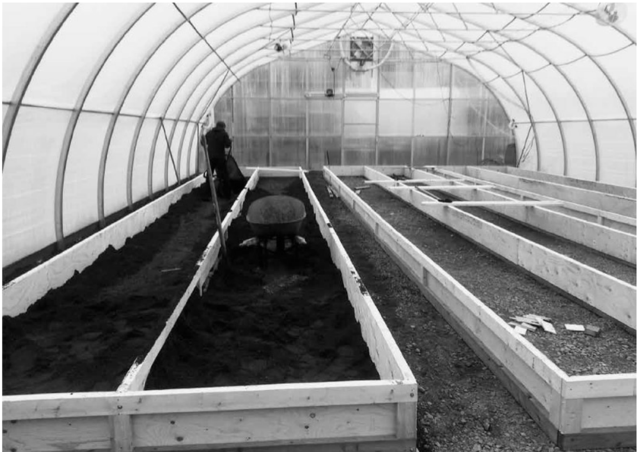
Laying the sand base in newly constructed troughs to protect the LDPE.
