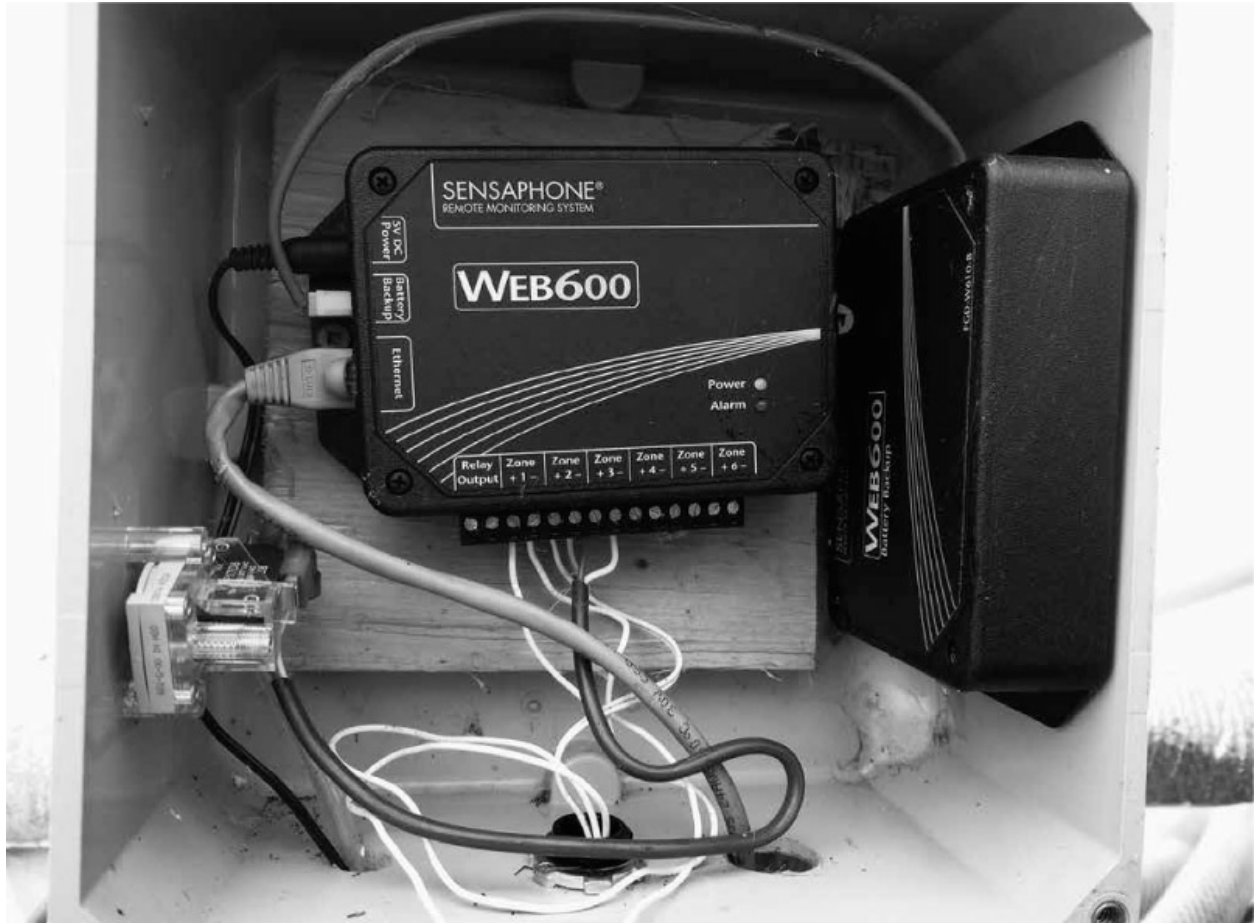
Web600 monitoring system with battery backup (right) and aeration pressure switch (left).
