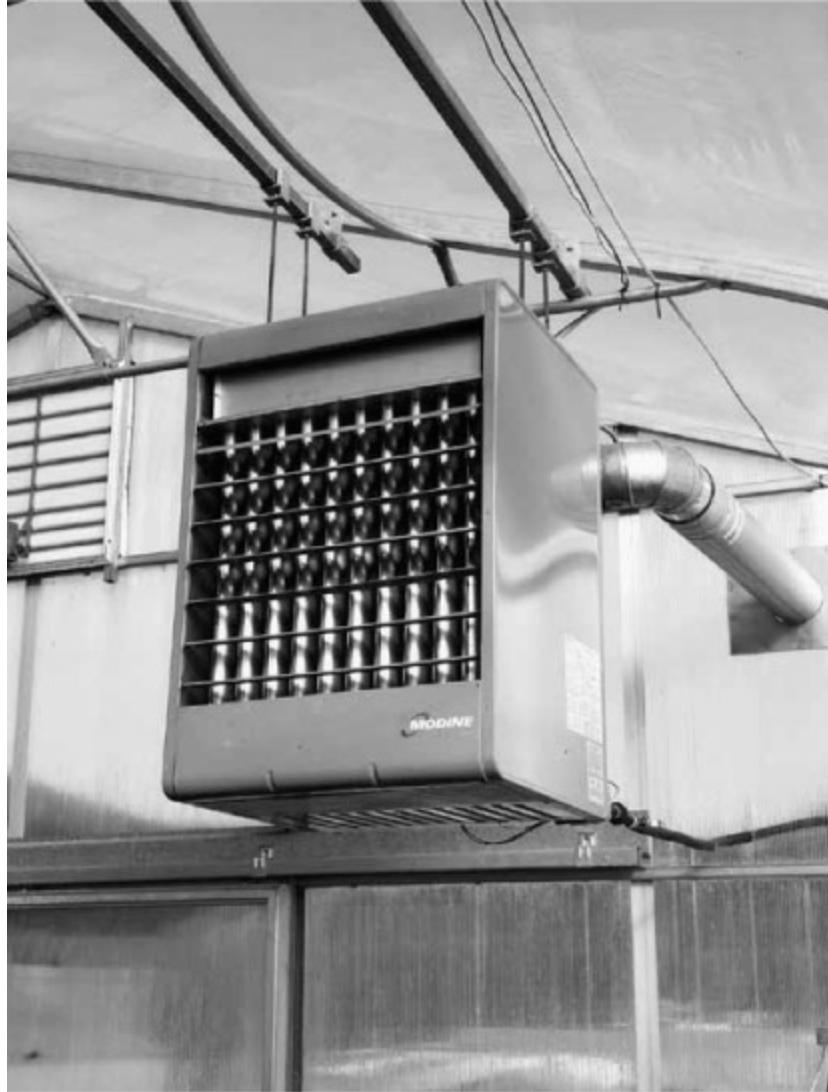
Vented propane greenhouse heater.
