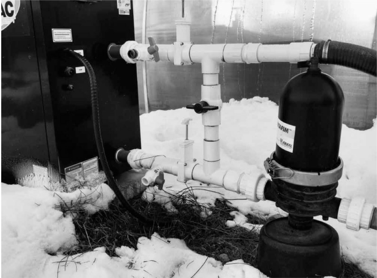
Heat pump bypass, inlet filter and flushing ports.
