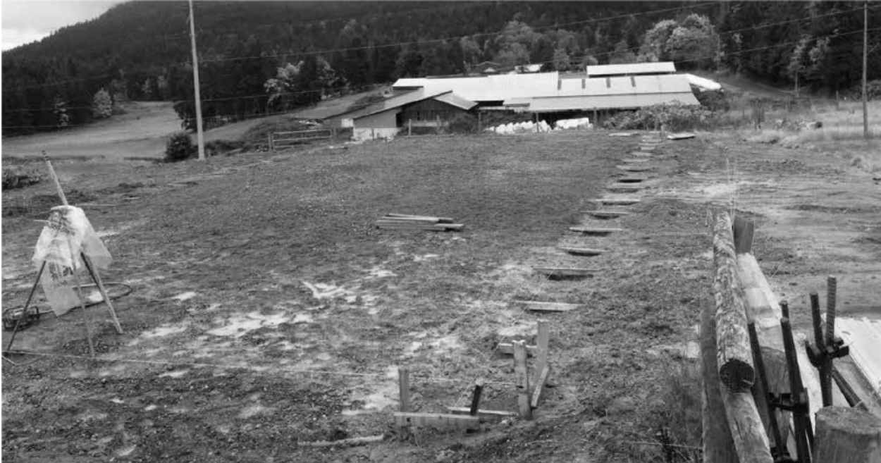
Foundation installation with string lines and batter boards, ready for concrete piers.
