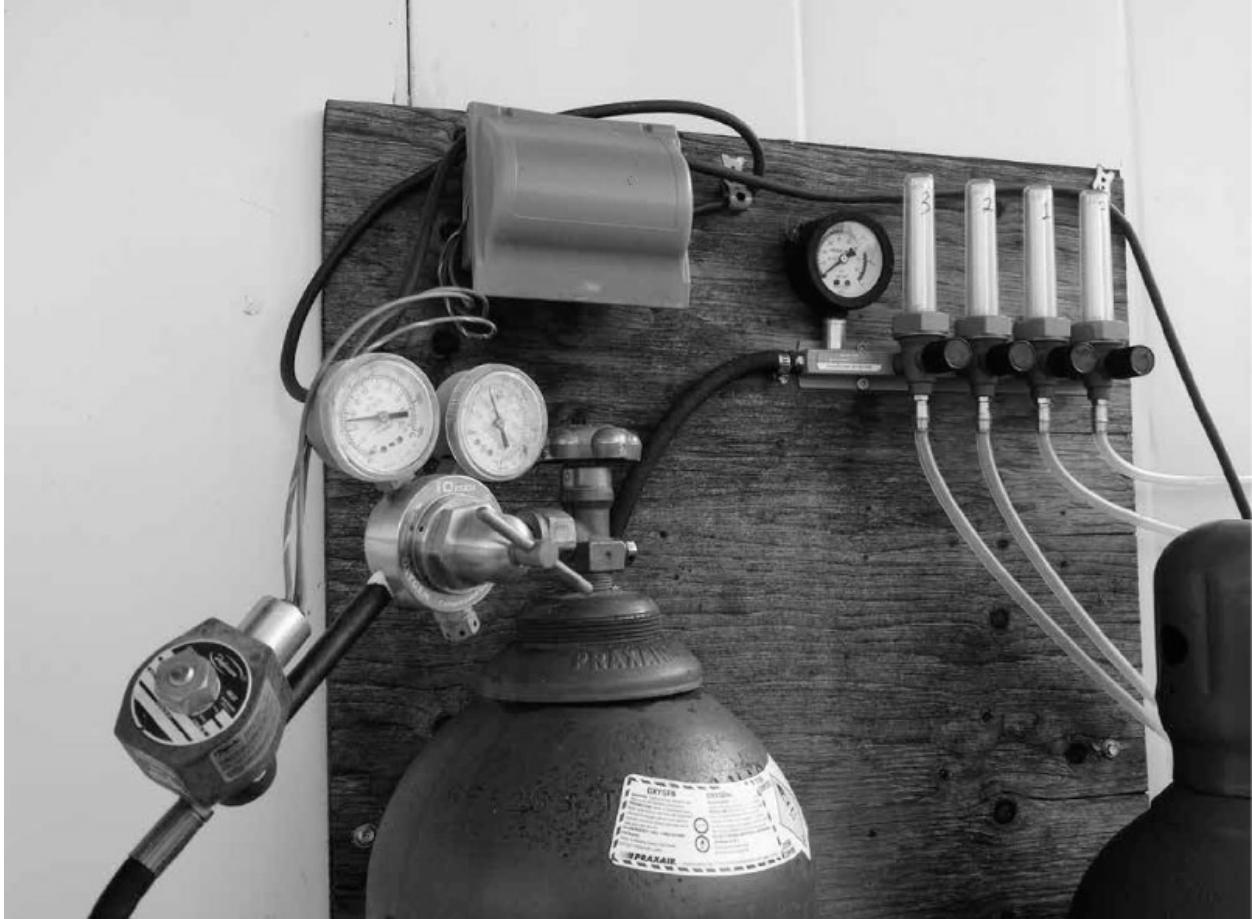
Backup oxygen system: oxygen tank, pressure regulator, solenoid valve and flow meter manifold.
