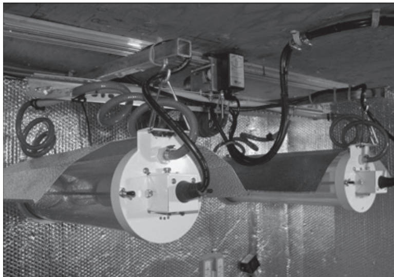
The HID lights in this indoor garden are water-cooled. The waste heat from the lights is used to heat the fish tank.
