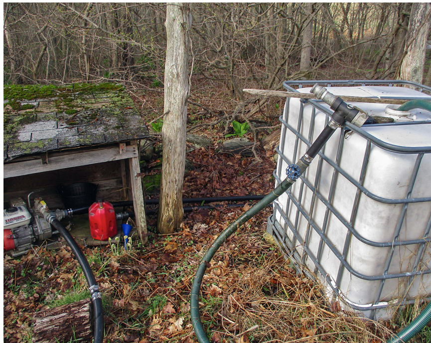
FIGURE 9.1. The line from the fertilizer tank can be inserted into our irrigation system's suction line using the quick-connection fittings. The valve on the fertilizer line adjusts the flow.
