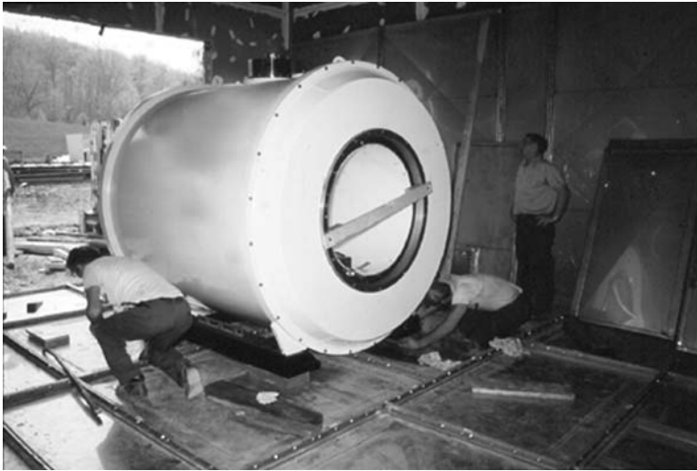
Figure 1.4 This is a picture of the 1.5 T superconducting magnet that was installed at Hershey-Penn State University Medical Center in 1985. This cylinder contains the superconducting wire and functions like a giant Dewar by providing thermal insulation for the liquid gases. Note the metal plates on the wall and floor that provide RF shielding for the scanner. This isolates the scanner from intruding radio waves that may be detected by the sensitive antenna and projected onto the image.
