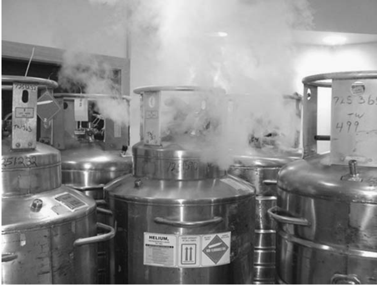
Figure 1.3 These many Dewars of liquid helium will be used to fill up the superconducting magnet of a 1.5 T MR scanner.
