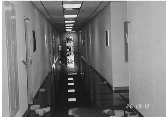
FIGURE 7.12 Two Inches of Water in a 20,000 Square Foot Facility is 25,000 Gallons.
