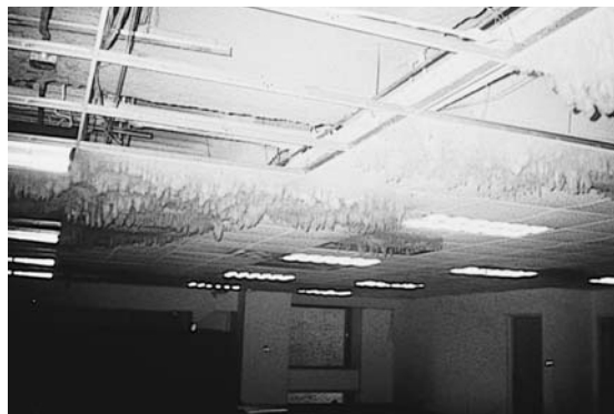
FIGURE 7.13 Fungus Growing on Water Saturated Ceiling Tile after Two Weeks Would Have Been Much Easier to Prevent Than to Clean.
