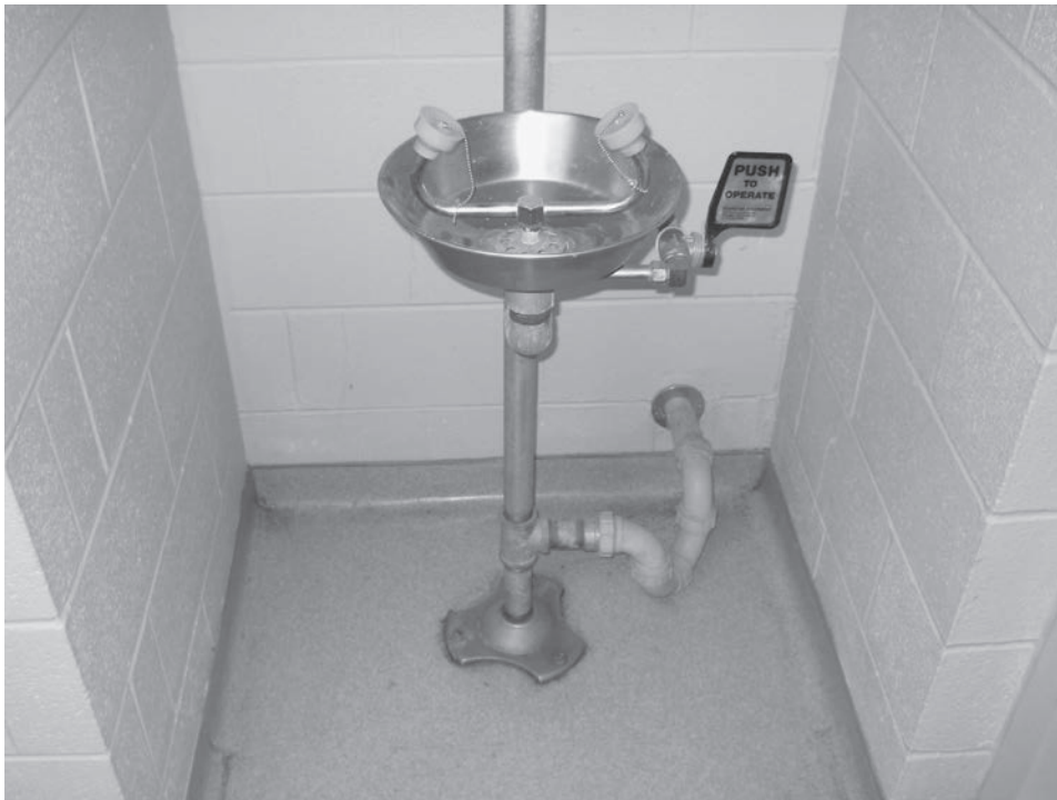
FIGURE 20–8 Emergency eyewash station.
