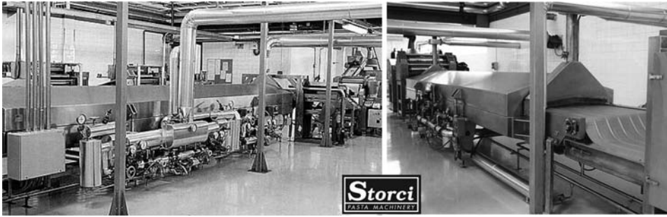
Figure 17.17 Pasteurization tunnel. (Courtesy of STORCI, Italy).
