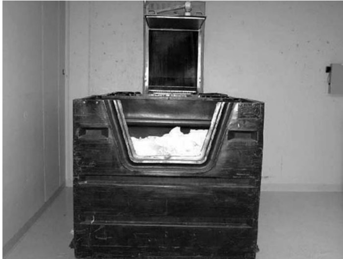
FIGURE 9.4 Trash chute discharge and receiving cart.
