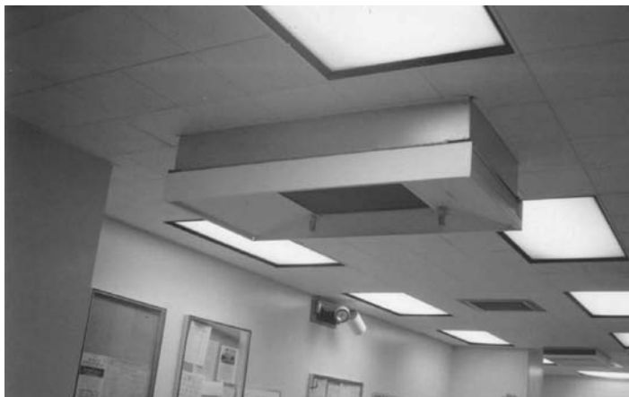
FIGURE 11.30 800 cfm ceiling-mounted HEPA unit.
