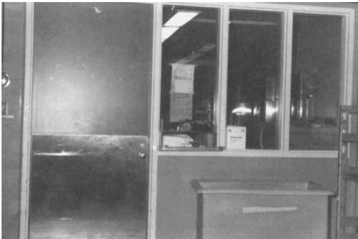
FIGURE 13.5 Separate EtO sterilizer room with 20 air changes per hour. (Photo by Frank Maniscalco.)
