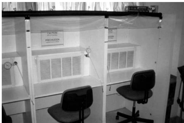
FIGURE 11.31 Built-in sputum-induction exhaust ventilation.
