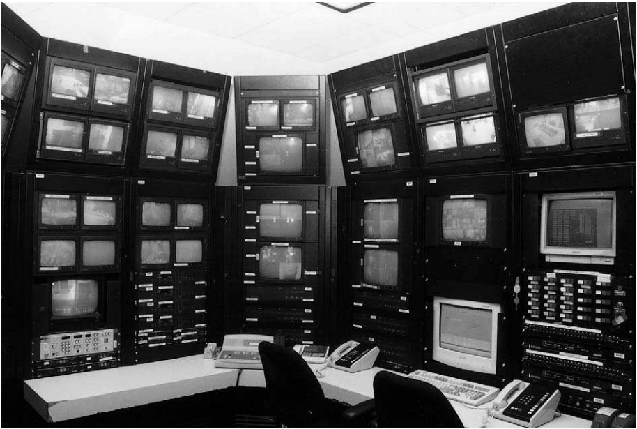
Figure 15-1 Example of a Central Security Station (Courtesy of New York University Medical Center Security Department)
