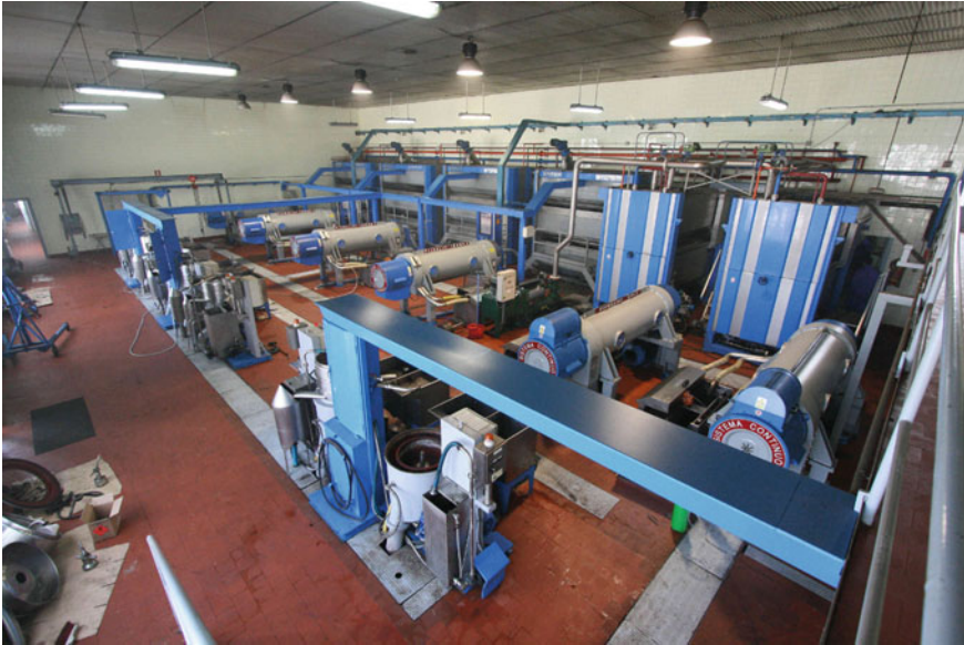
Fig. 6.1 Picture of an industrial olive oil production plant
