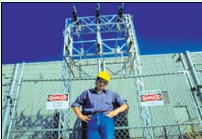
This exposed electrical equipment is guarded by an 8-foot fence.
