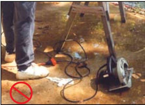
Combinations of hazards increase risk.
