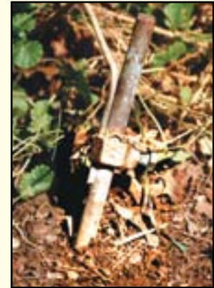
Grounding rod in the earth.
