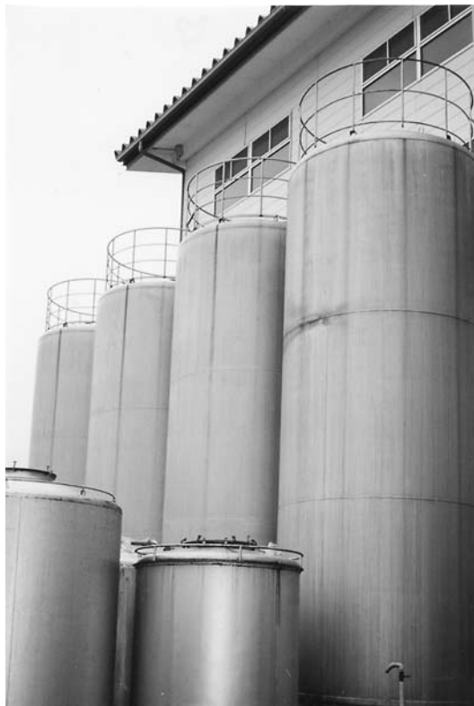
Figure 20 At some modern factories, the large-scale fermentation tanks and the storage tanks are installed outdoors.
