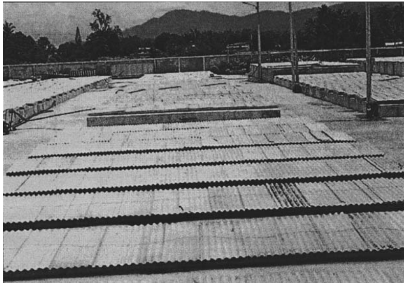
Figure 5 Outdoor concrete pools for fish sauce production in a large factory. (Courtesy of Pichai Fish Sauce Co., Ltd.)
